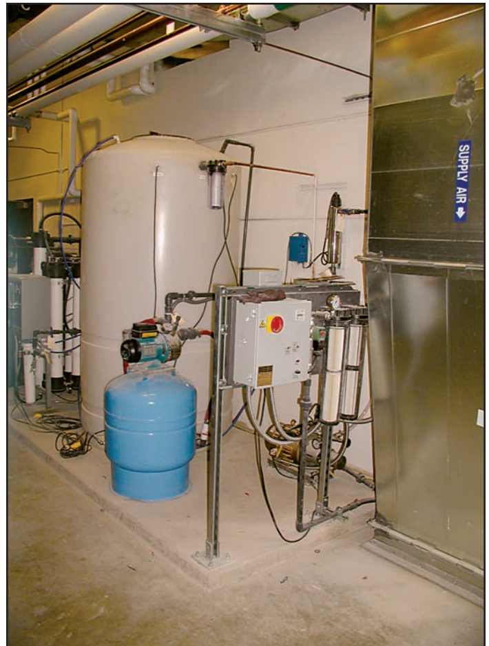
The water treatment system at NSF consists of pre-treatment carbon and water softeners, an RO system, water storage and re-pressurization, and water sterilization UV unit on the system discharge. All adiabatic humidification systems require water treatment to remove dissolved minerals and solids.
