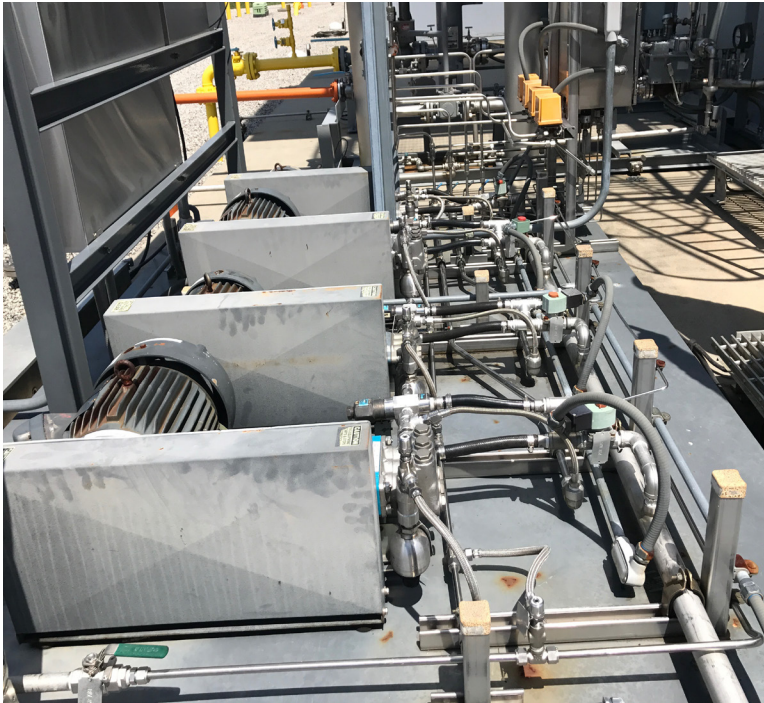
MeeFog Skid before upgrade
