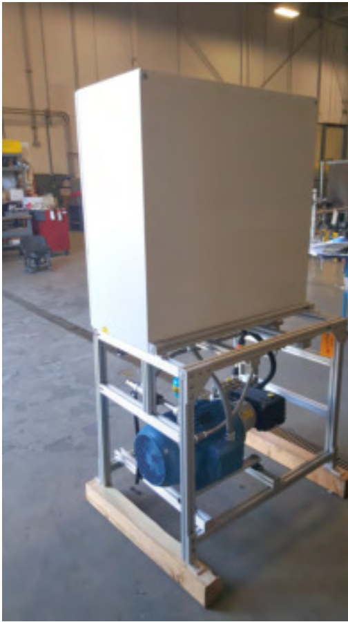
Pump rack 1 before installation
