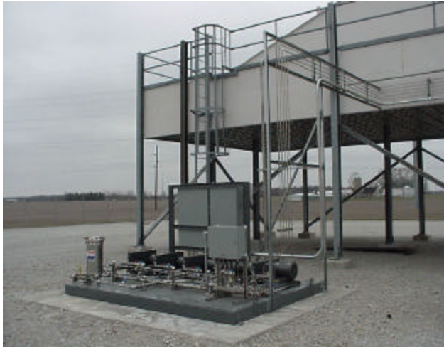
Figure 2. Typical high pressure fogging skid. The feed lines from the high pressure pumps to the inlet system can be seen here.
