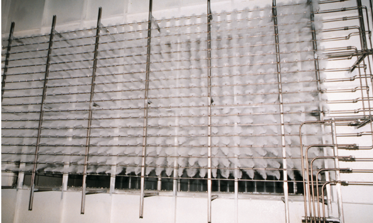
Fog Lines staged for precise control in air plenum.
