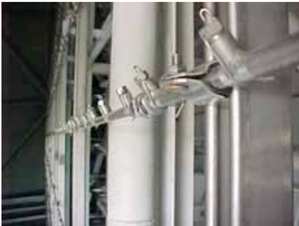
Figure 6. Individual nozzle line showing fog nozzles.
