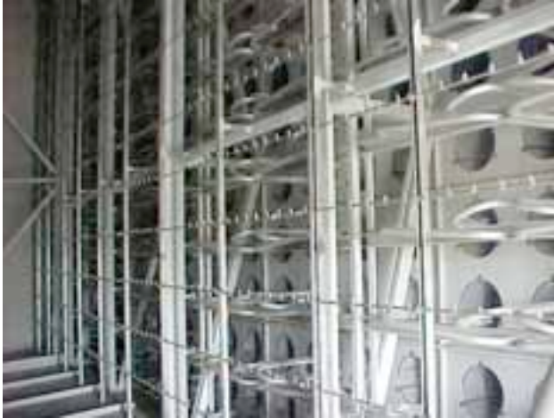
Figure 5. Fog Nozzle Manifold after the inlet filters
