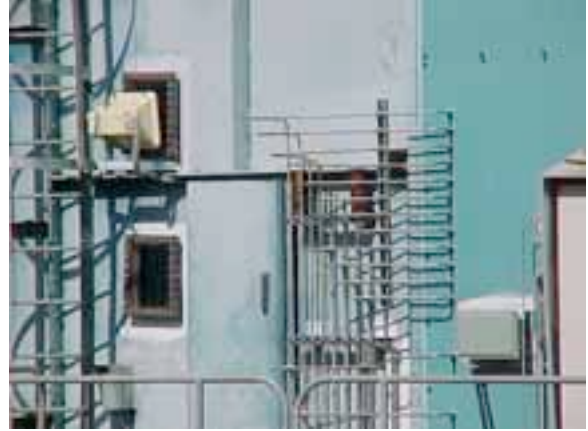
Figure 9. Penetration of high pressure fogging tubing into the inlet duct for the multiple cooling stages. The viewing window can be seen to the left. The upper window is to provide lighting.
