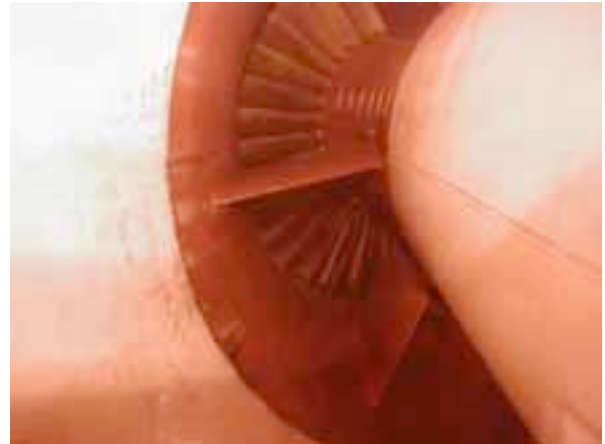
Figure 10. View from compressor inlet plenum viewing window.
