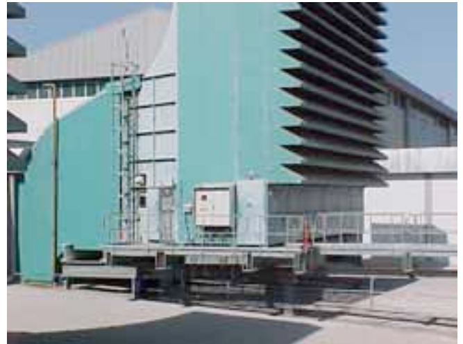
Figure 8. Inlet duct of the gas turbine. The interconnecting pipes can be seen under the walkway.
