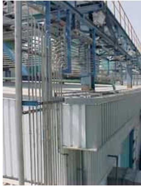
Figure 7. Interconnecting Piping from the skids to the gas turbine.
