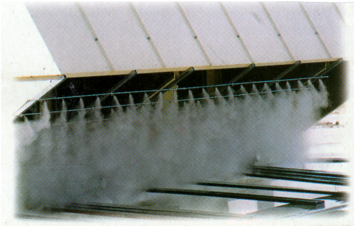
Figure 2. Fog Nozzles in operation upstream of Filters.
