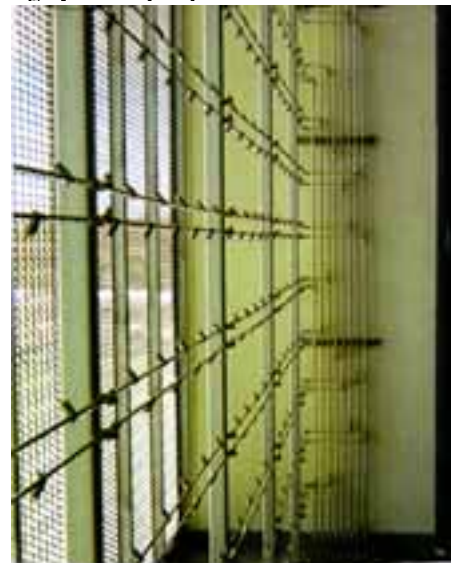
Figure 10. High Pressure Fog Manifold.
