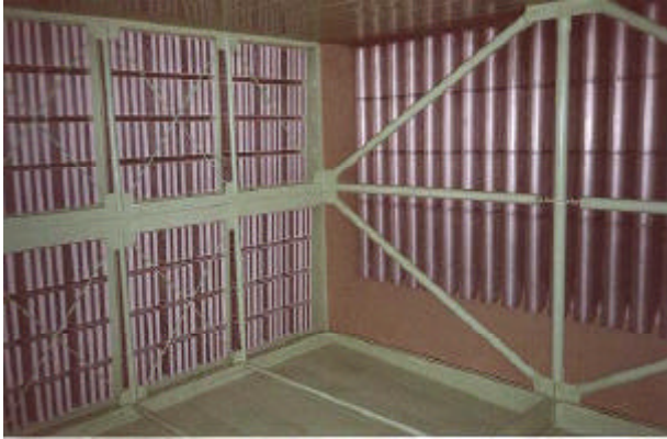
Figure 8. Typical obstruction found in an inlet air duct
