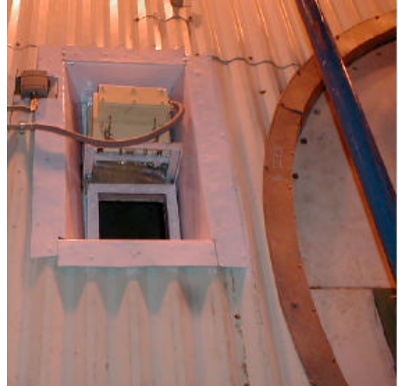
Figure 28. Viewing window at the compressor inlet section of a large gas turbine. Upper window is for lighting arrangement
