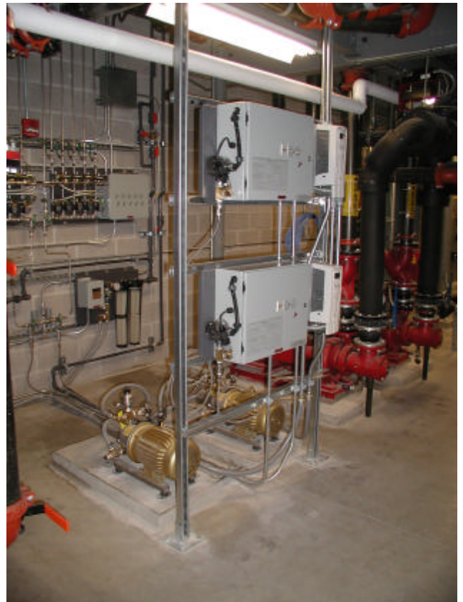
Mee Fog Dual Pump System Installation
