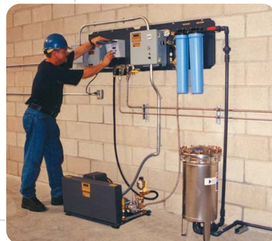
Typical Mee Fog system pump station.
