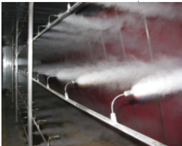
Fog manifolds run independently to stage the amount of humidification supplied.
