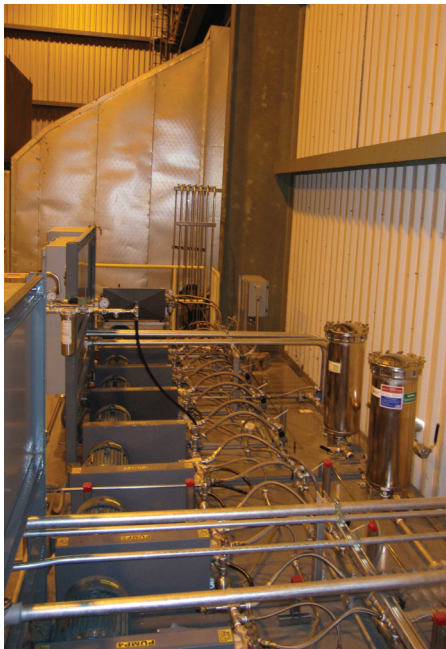
Figure 2: A Mee fog skid at Midland Cogeneration
