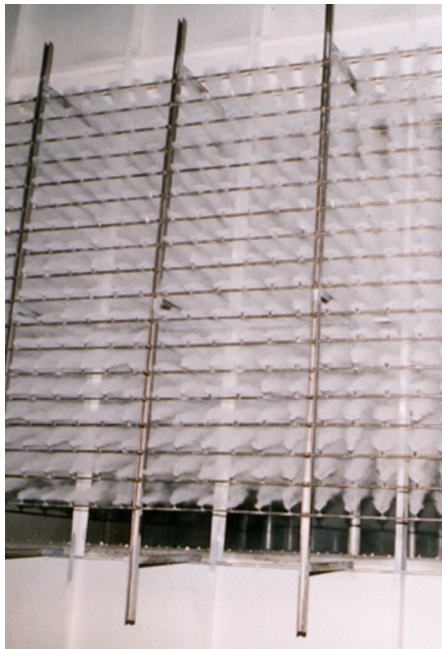
Figure 3: Fog array at the gas turbine inlet
