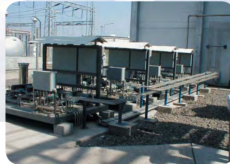
Turnkey installation at a 600 MW combined cycle power plant. This project involved six MeeFog™ skids and the turnkey installation of 2.5 km of high-pressure tubing, fog system commissioning, and start-up.
