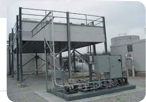
The high-pressure MeeFog™ skid is reliable and carefully engineered. MeeFog™ skids have been supplied to several major utilities and GT OEMs with a large number of repeat orders. Installations can be done with only a 1-2 day outage.
