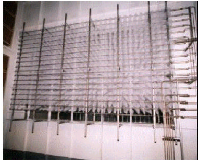
Fig 2. Fogging nozzle array showing nozzles in operation
