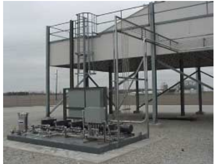
Figure 2. Typical high pressure fogging skid. The feed lines from the high pressure pumps to the inlet system can be seen here.
